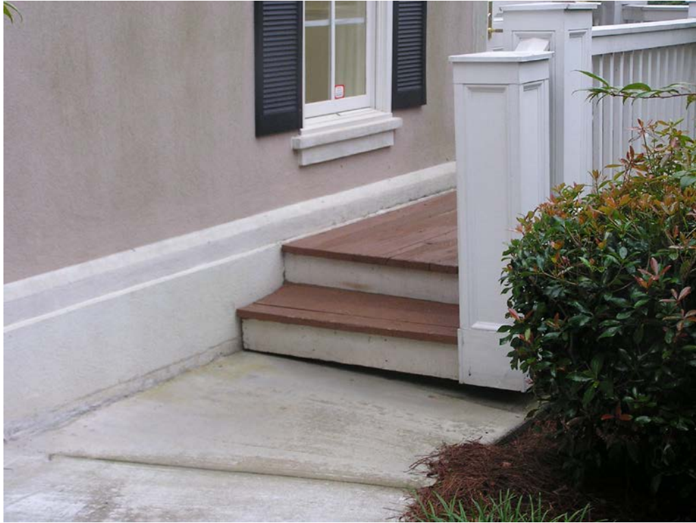
23. Collapsed wood step located at the right side of the clubhouse.
