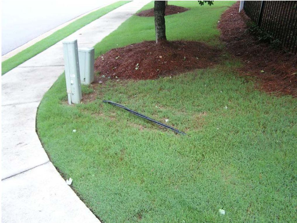
30. Exposed electrical cable at the sidewalk located near the left front side of the clubhouse.
