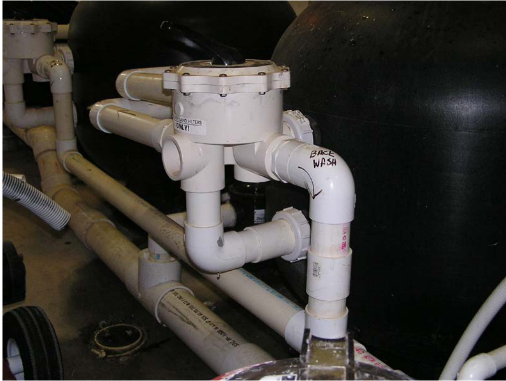
39. View showing the leaking valve at the filtration equipment for the main pool.
