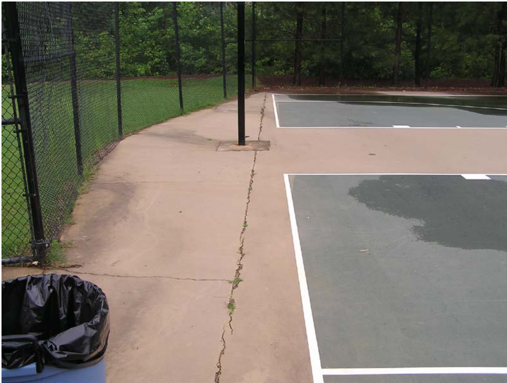
12. Deteriorated cold joints in the asphalt surface of the basketball court.
