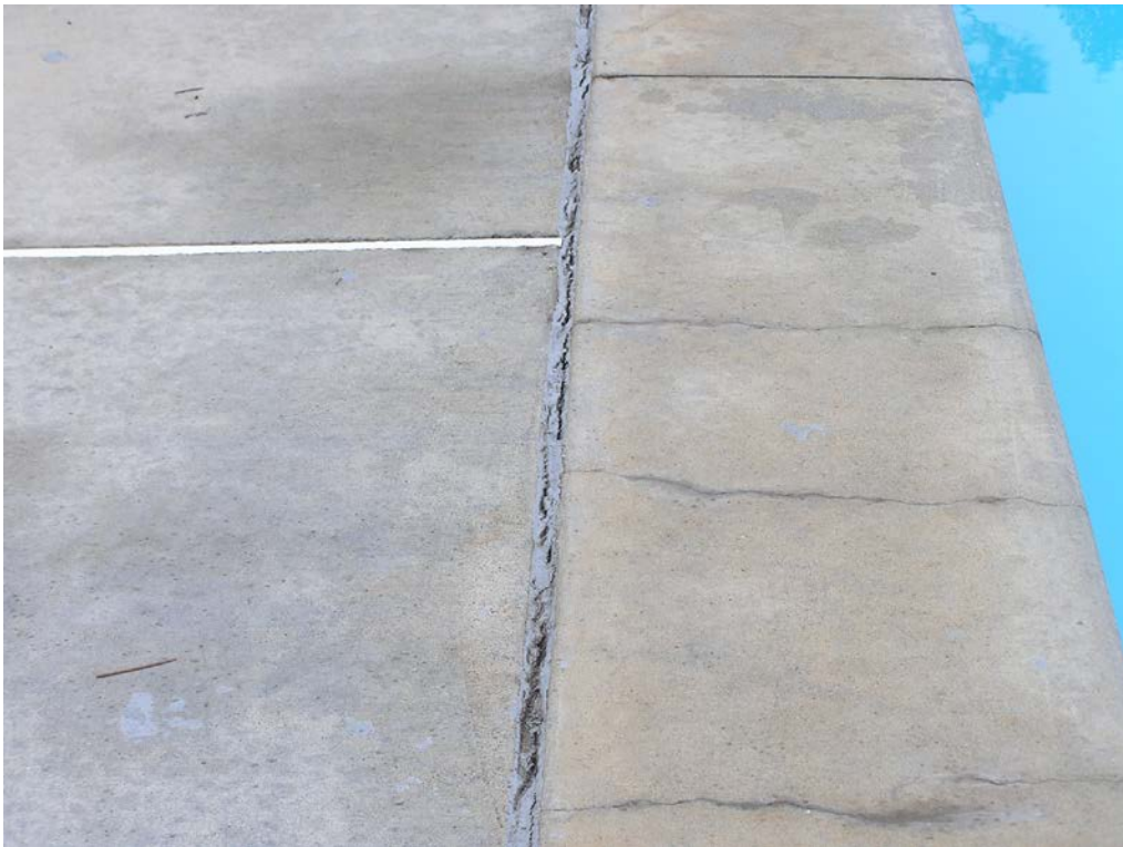
6. Deteriorated caulk joint at the main pool.
