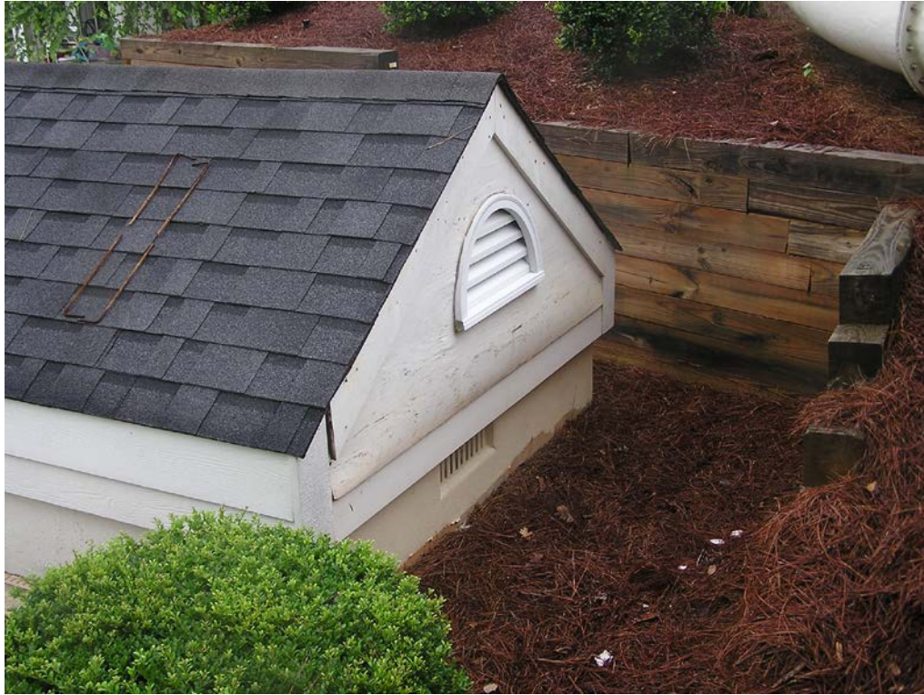
29. Deteriorated wood access panel at the waterslide pump house.
