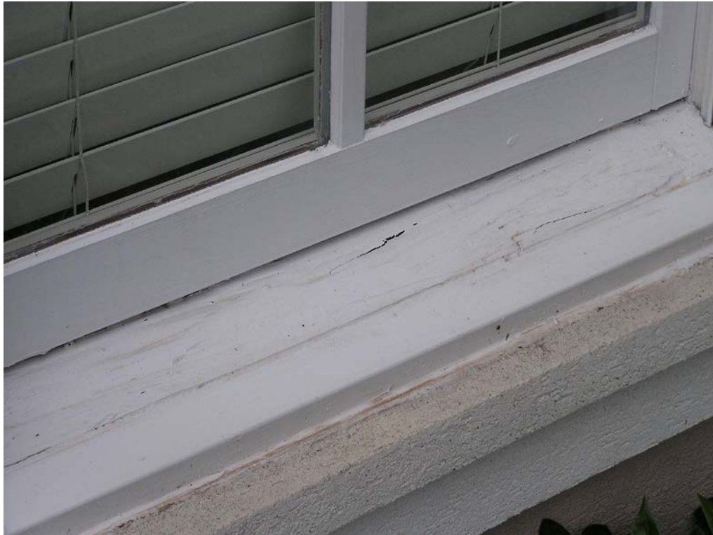
24. Deteriorated wood windowsill at the right front side of the clubhouse.
