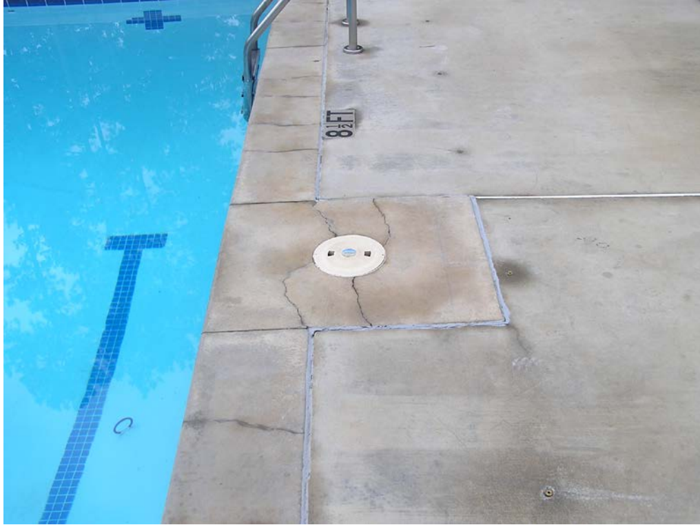
7. Cracks in the concrete deck at a typical skimmer opening at the main pool.
