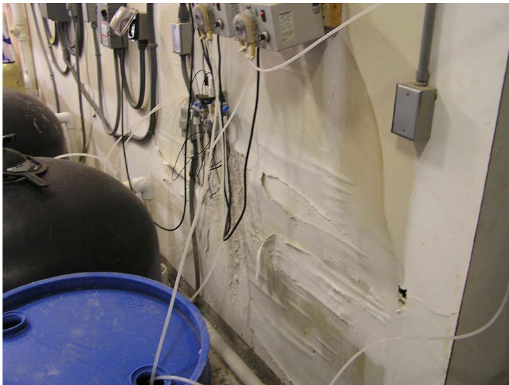
36. Deteriorated gypsum board walls in the pool equipment room.
