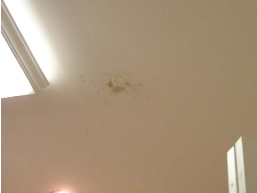
31. View of the kitchen ceiling showing mildew stains, indicating a possible leak problem.
