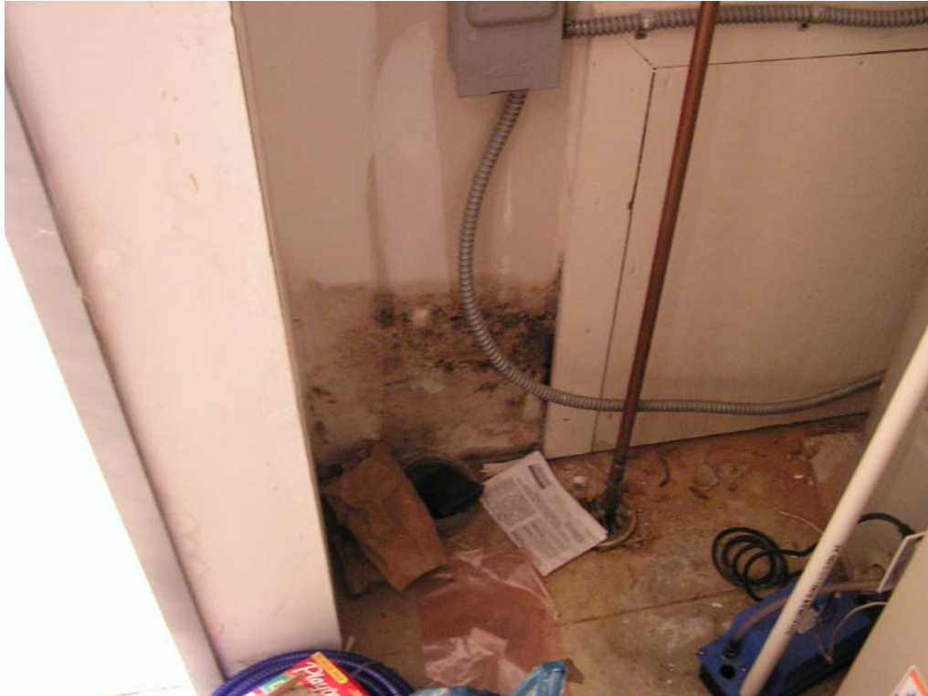
35. View showing deteriorated and mildew-stained gypsum board walls at the lower level mechanical room, indicating a possible plumbing leak problem.
