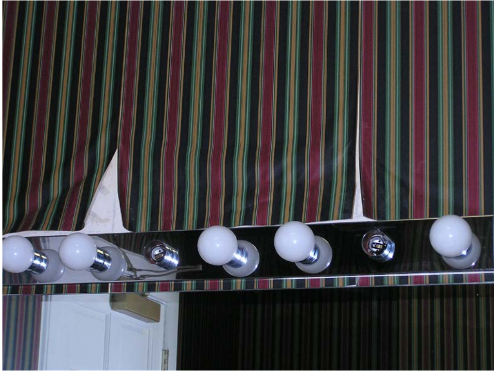
33. View showing peeling wallpaper in the upper level men's restroom.
