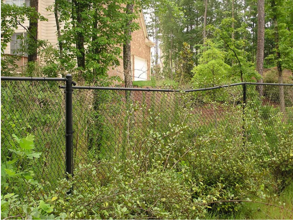
5. Damaged chain link fence at the detention pond adjacent to 5425 Stone Croft Trail.
