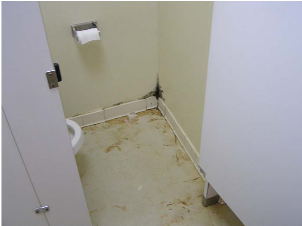
34. View showing deteriorated and mildew-stained gypsum board walls at the lower level men's restroom, indicating a possible foundation leak problem.
