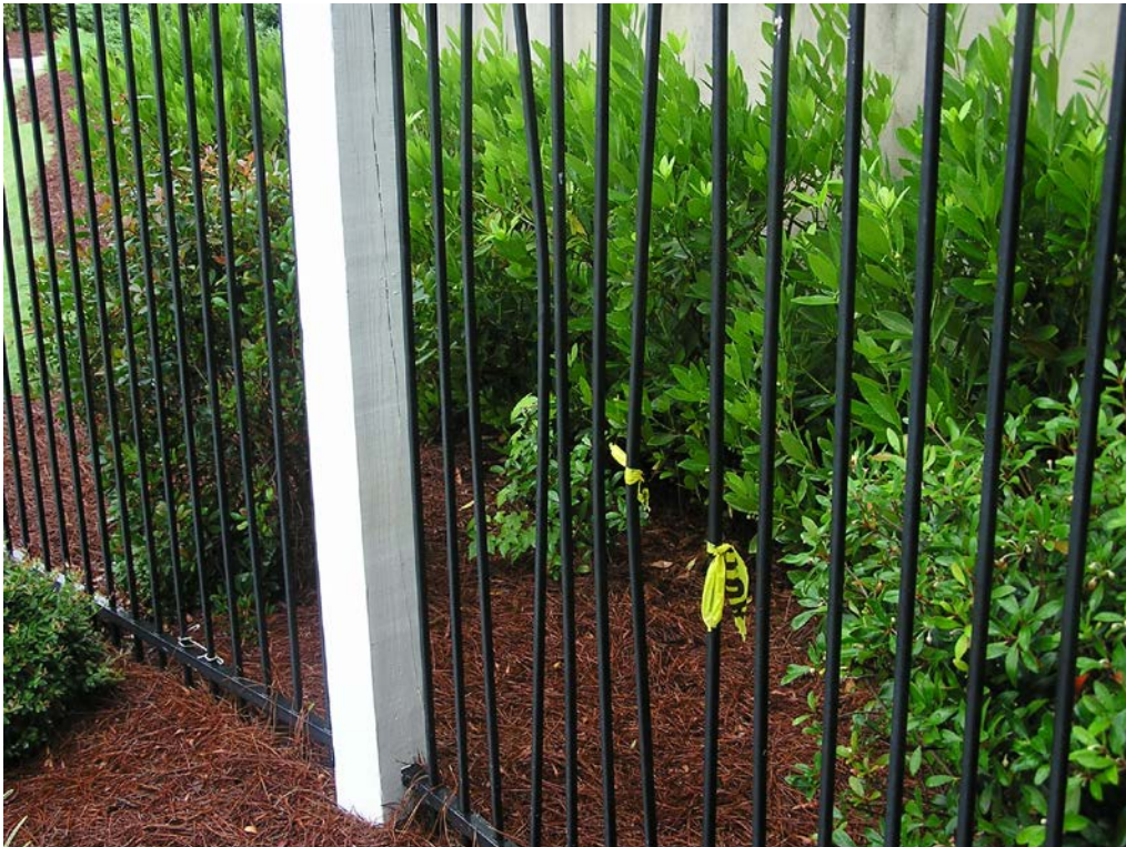
10. Typical damaged aluminum fence pickets at the perimeter fence surrounding the pool deck.
