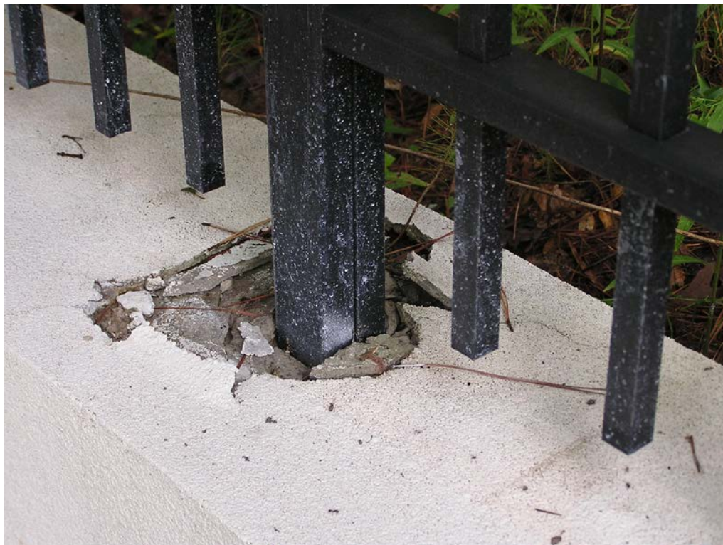
4. View showing a loose fence post and deteriorated stucco finish at the wall paralleling the main entry drive.
