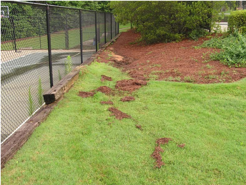
14. General view showing evidence of poor drainage and erosion occurring at the top of the retaining wall at the basketball court.
