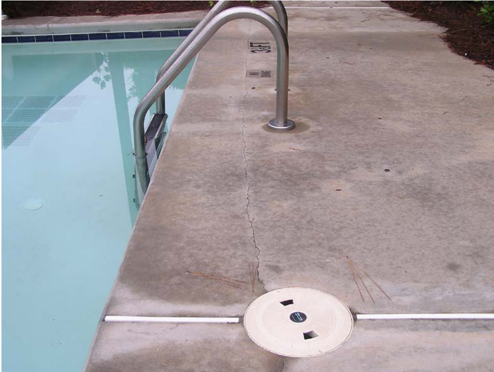
9. Hairline crack at the waterslide pool that appears to have occurred due to slight settlement.
