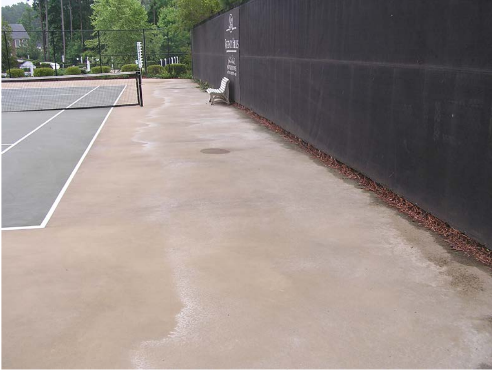
13. View showing evidence of ponding water at the south side of the tennis courts.
