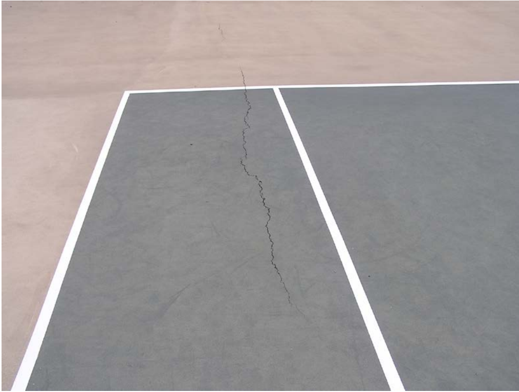
11. View showing typical cracks in the asphalt wearing course of the tennis courts.
